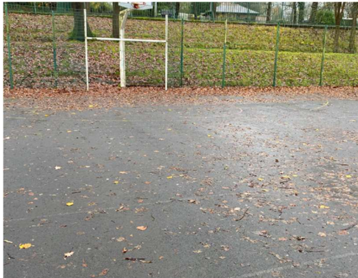
Faded line markings
