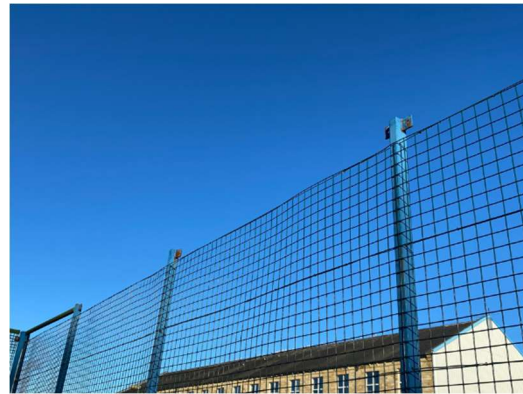
Top rails on fence missing
