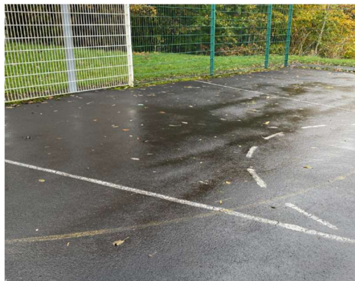
Faded line markings
