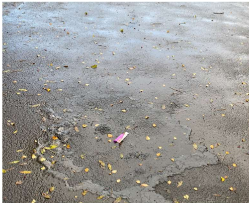
Damaged MUGA surface
