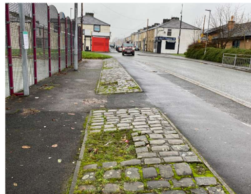
Voids at former tree pits/missing setts
