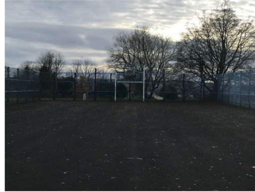
Faded line markings
