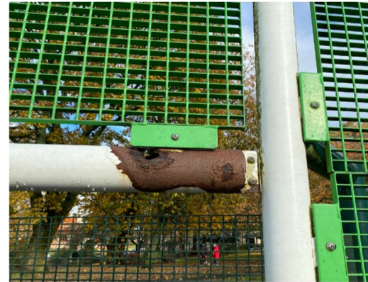
Rusted goal post at fixing
