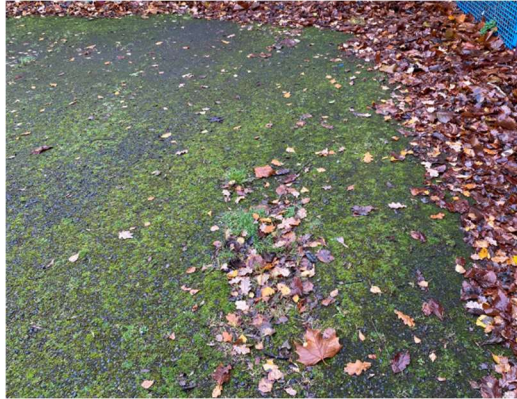
MUGA surface in poor condition
