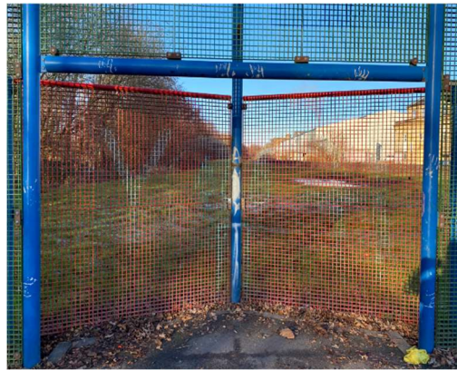
Scuffs/paint missing on goal posts
