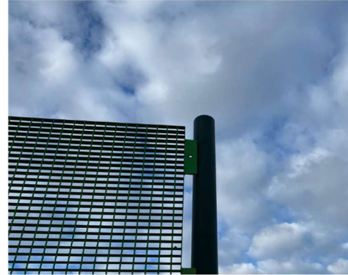
4 No. bolts missing on fence
