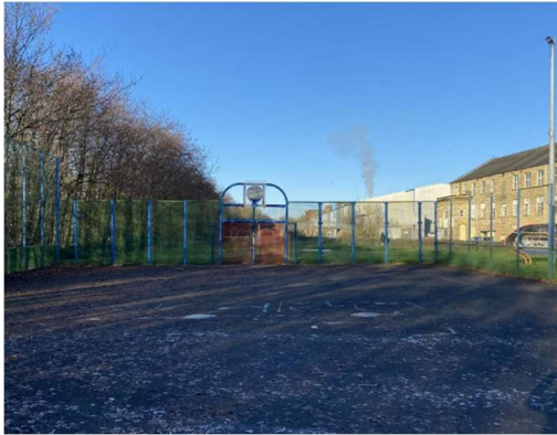
Faded line markings
