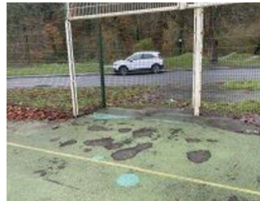
MUGA surface in poor condition
