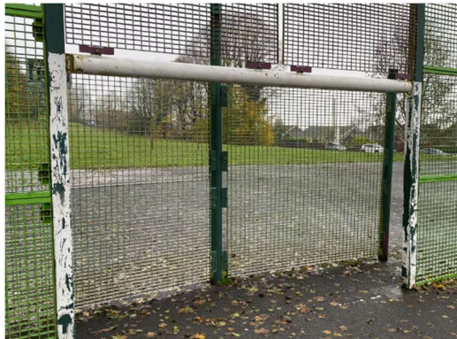
Rusted/scuffed goal posts
