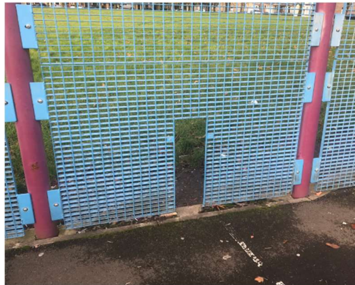
Cricket wicket missing from fence
