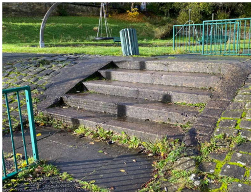
Steps restrict disabled access
