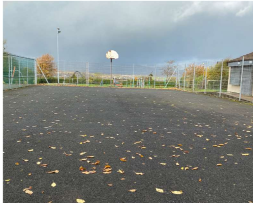
Faded line markings
