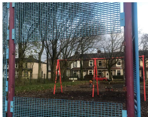
Missing fence panel
