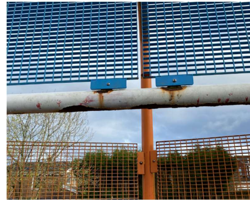
Goal posts have rusted
