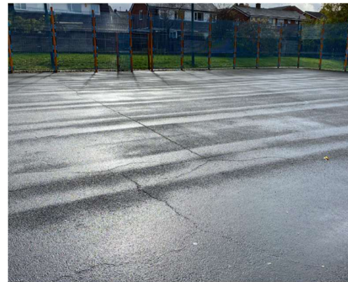
Cracks in MUGA surface
