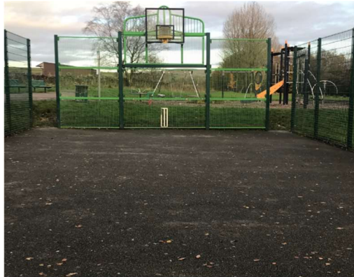
Faded line markings
