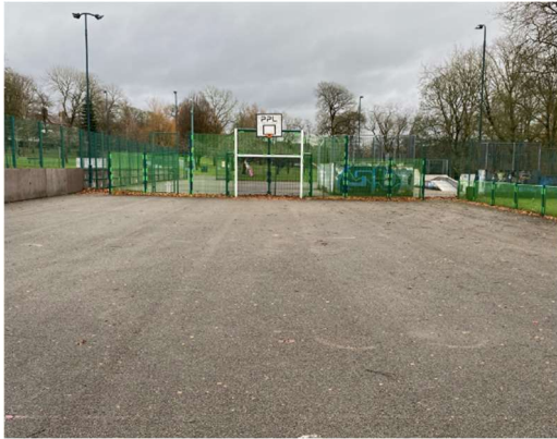
Faded line markings
