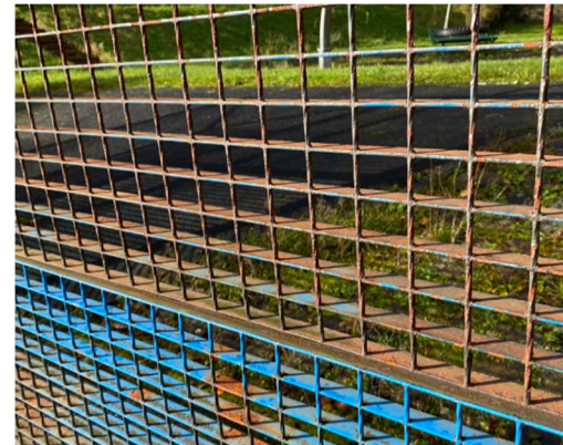
Fence is rusted
