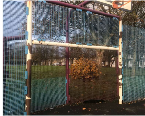
Rusted goal posts
