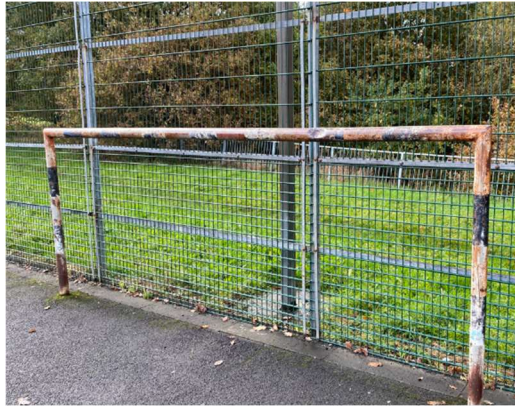
Rusted goal posts
