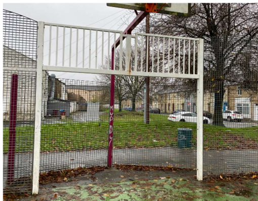
Graffitied/faded paint on goal posts
