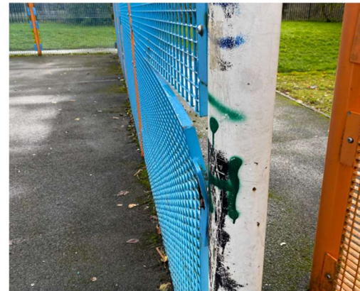
Fence panel bent outwards
