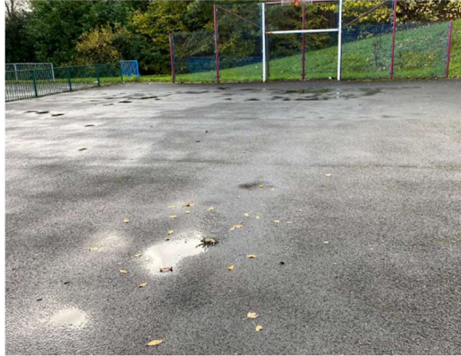
Faded line markings
