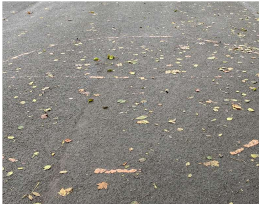
Faded line markings
