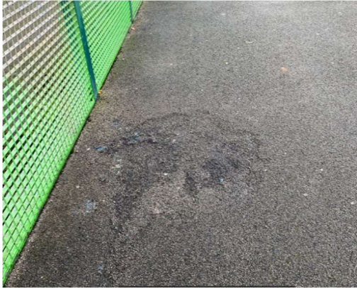
Damaged MUGA surface
