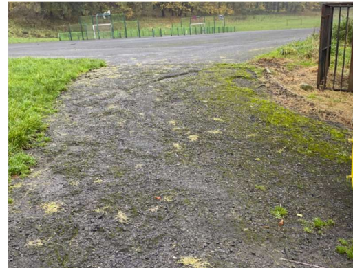
Footpath connection in poor condition
