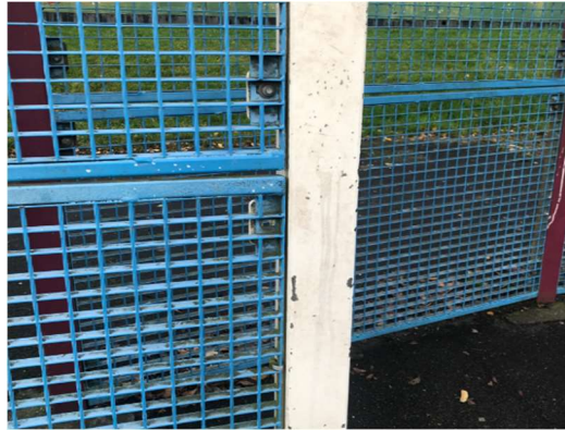
Bolt missing in fence
