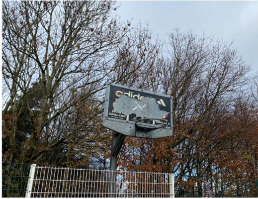
Damaged basketball backboards
