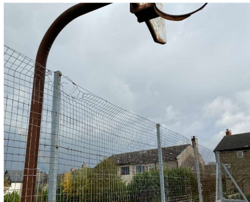
Sections of fence in poor condition
