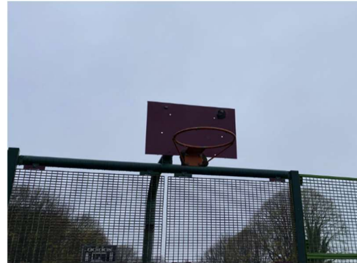
Damaged basketball backboard
