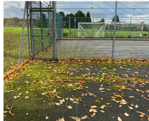
MUGA surface in poor condition
