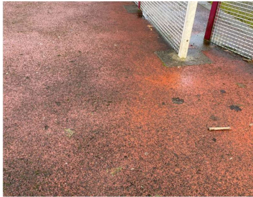
MUGA surface in poor condition
