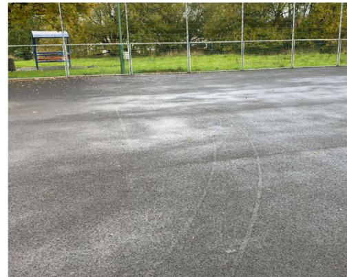
Faded line markings
