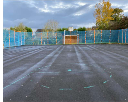
Faded line markings
